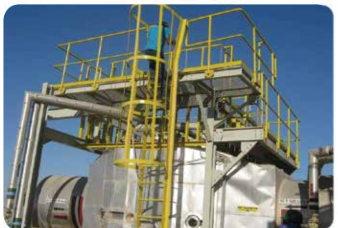
Mist Eliminator Platform
