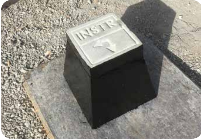
Cable Route Marker
